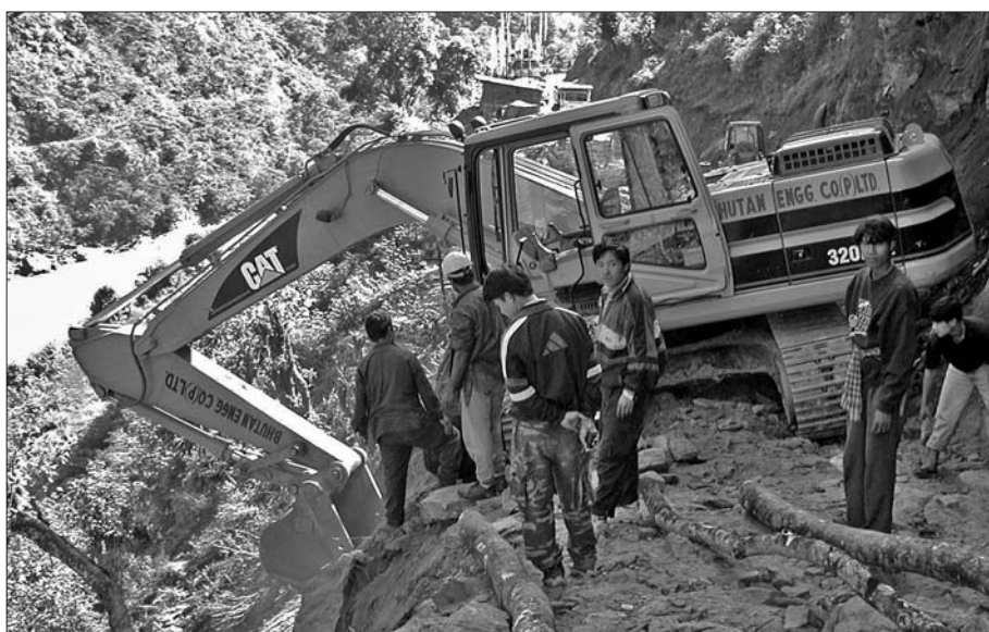
Photo: SNV 'Bulldozers have been replaced by excavators, which allows for the loading of tippers and the transport of excavated surplus material and debris to selected spoil disposal sites.'
